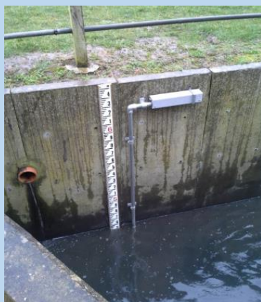
Figure 7-4 Water level monitoring installation in Peterborough
