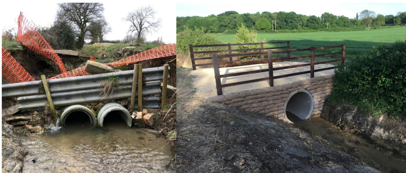
Figure 7-3 Culvert collapse and subsequent on Marholm Brook
